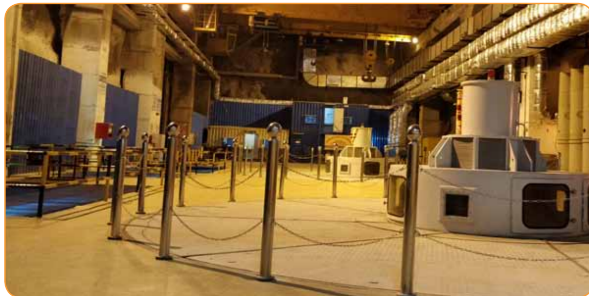
Turbine Generator - Dikchu HEP
