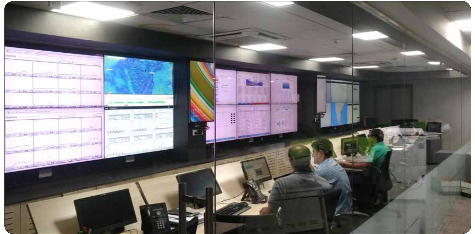
Real time monitoring of Greenko Assets by Centralized SCADA System
